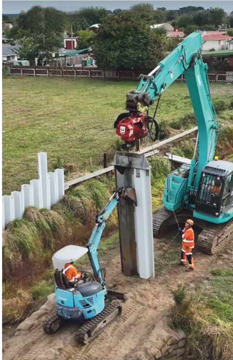
Diggers lift sheetpiling to install on the opposite bank of Kings Canal Drain in Foxton. Photo Horizons Regional Council
